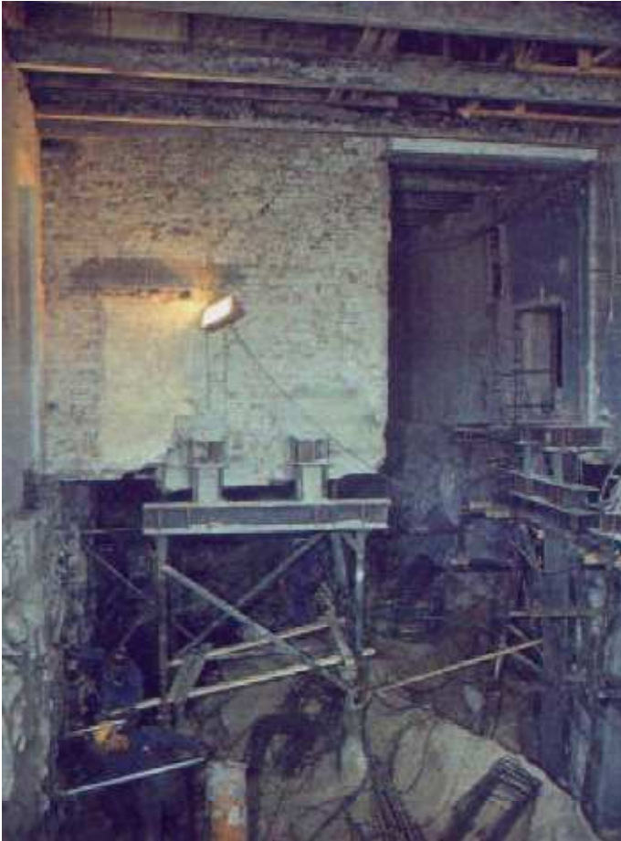
Photograph 4. On the right: middle wall. Center: reinforced concrete column and temporary steel supports, braced steel pile truss. Left: injection work (northern wall).
