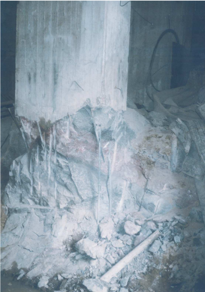
Photograph 6. Eastern stair column. Structural stages. Loosened, fissured rock. Dowels and hammer visible.
