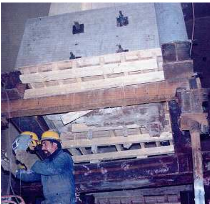
Photograph 5. Eastern stair column. Structural stages. Old brick column. Pretensioned concrete plates. Temporary steel supports.
