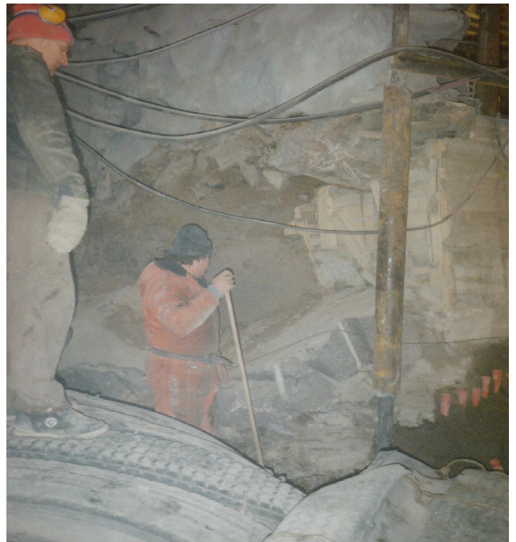
Photograph 3. Middle wall. Drilled steel piles. Smooth blasted face. Close spaced holes ready for old hand method loosening rock with hammer and wedges.
