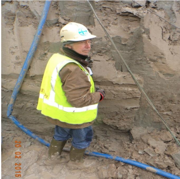
Figure 14. Test trench, depth of visible crack apr. 1,8m from surface.
