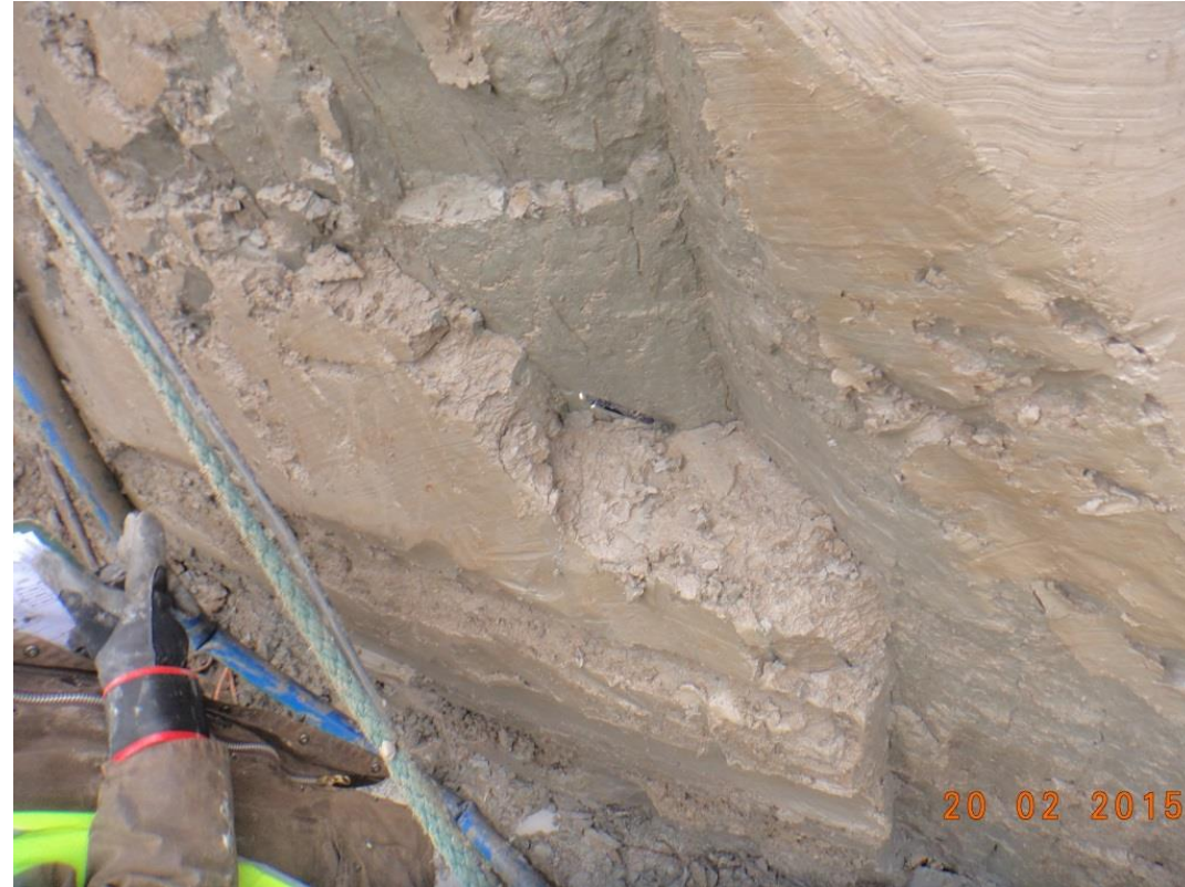
Figure 15. Detail picture of the crack.
